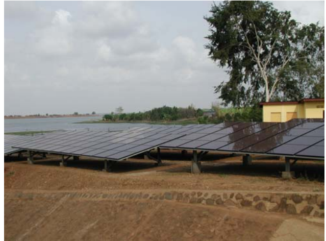
Solar System Project in Kampong Cham Province
