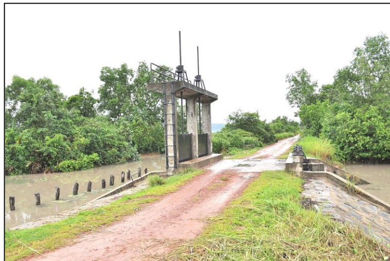
Figure 5: Regulator for control of drainage, flooding and saline intrusion, Sameakki Commune
