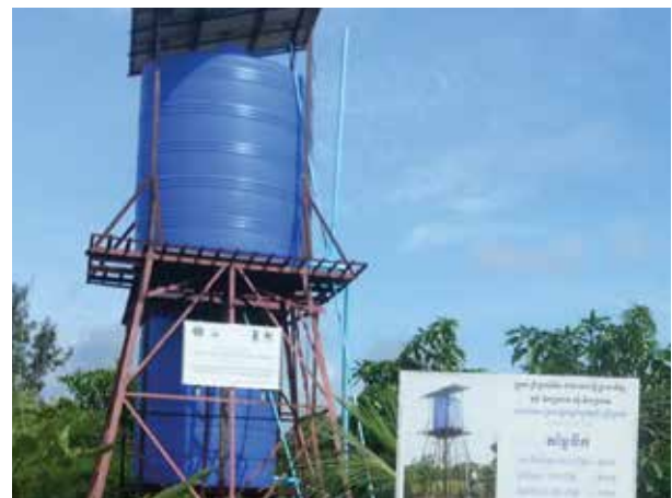
Solar water pumping system in Bos leav commune, Kracheh province
