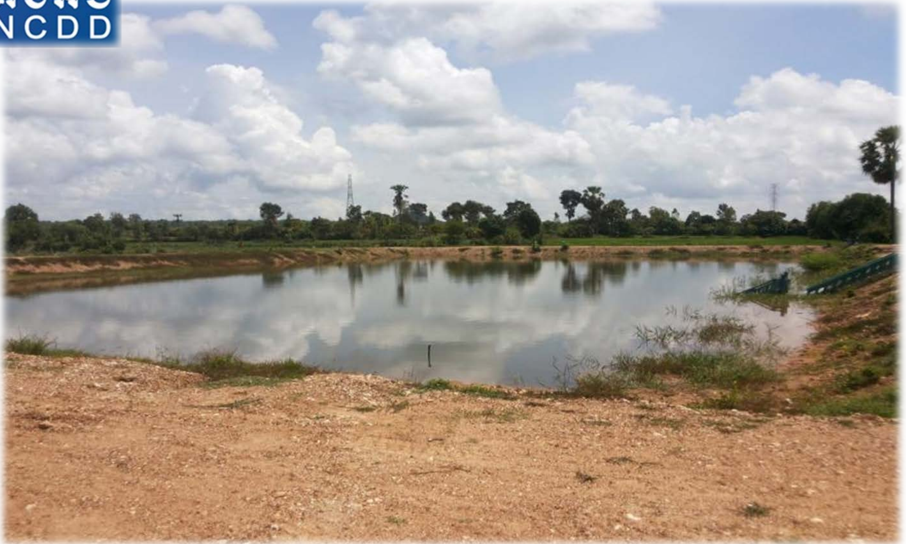
Lumpong commune: a pond rehabilitated, size 60m x 34m x 2m, total budget Khmer Riels 15,300,000 with 0% contribution from commune fund and 100% from LGCC. The project was implemented from 15 th November 2012 to December 2012. Picture taken in October 2013.
