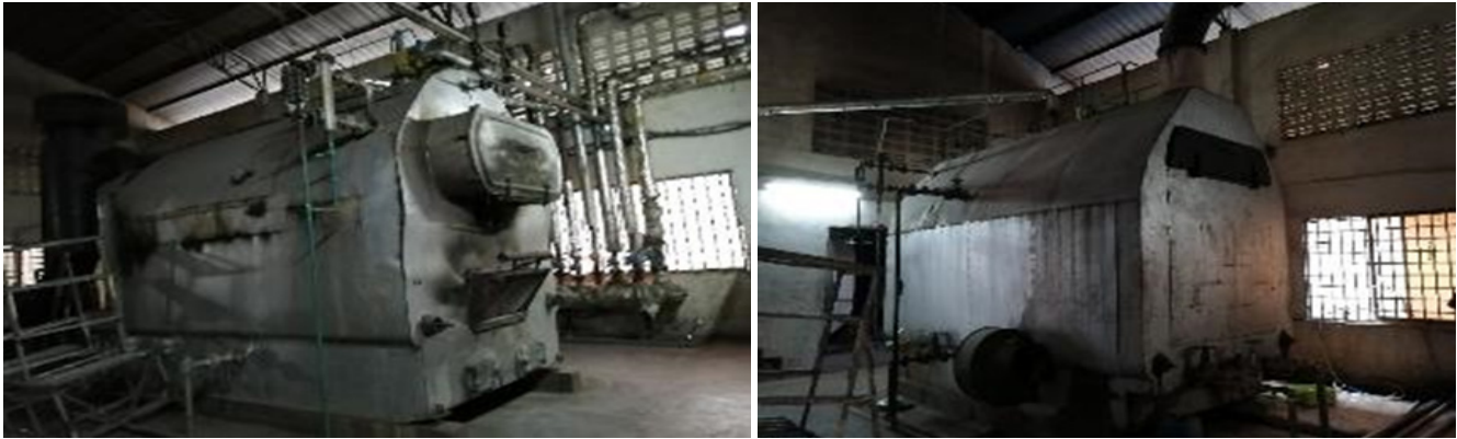
Figure 4: Two backup fire-tube boilers (2 TPH)
