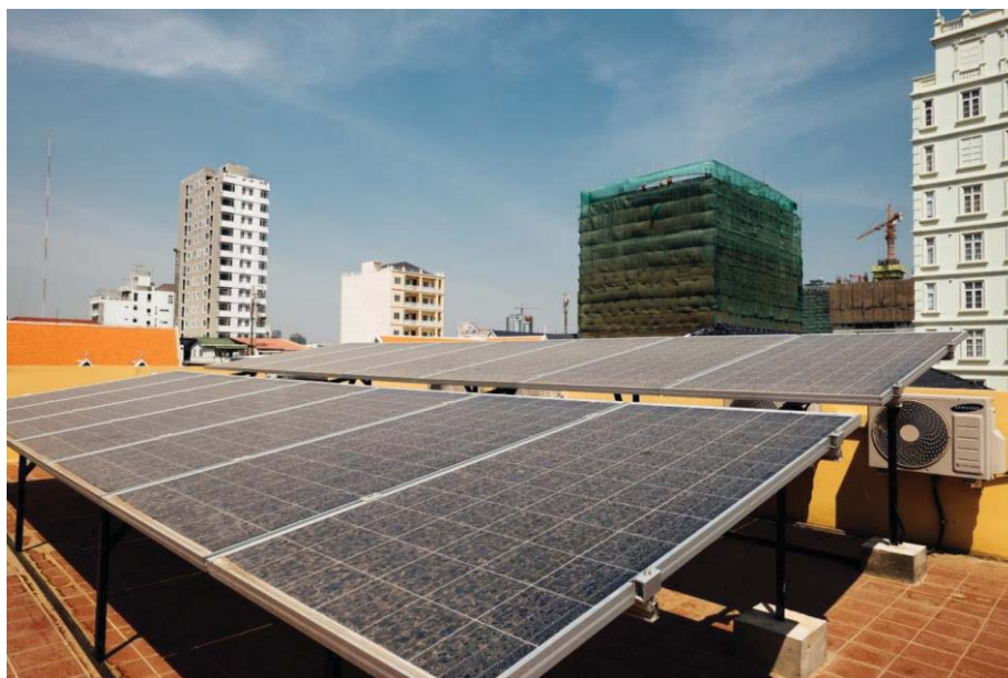
Figure 10. There is substantial potential for roof-top solar PV in Phnom Penh to service households, businesses and manufacturing (photograph by Bernardo Salce).
