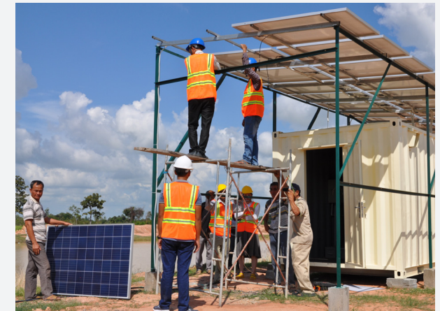
Installations of Solar Power Station for household micro grid, Sep 2018, Pursat province
