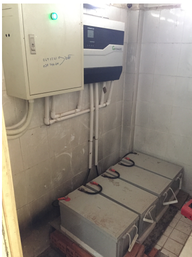
The 2.5 kWp and 10 kWh solar-powered battery system installed at the health center
