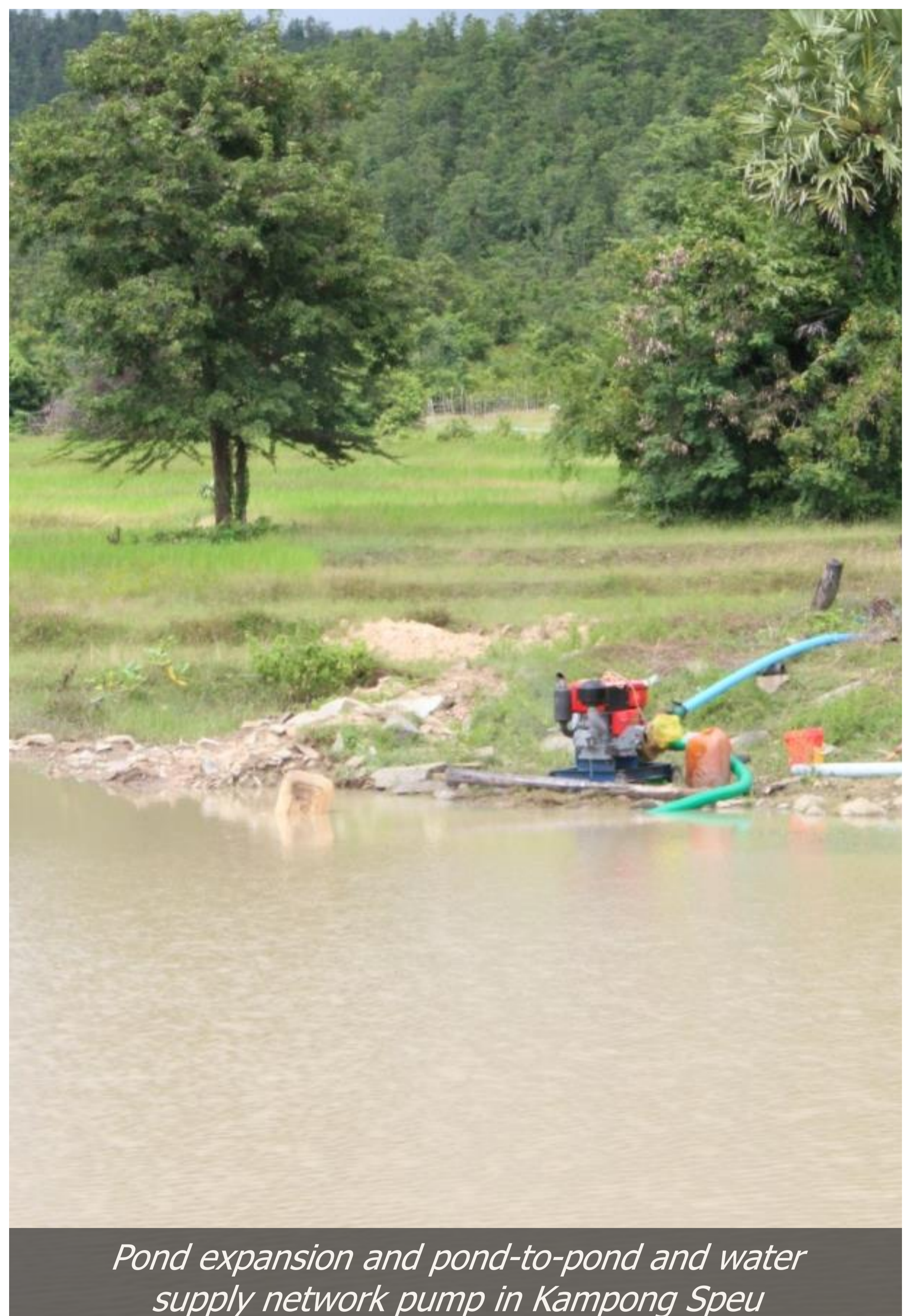
Water supply system construction at Tbong Kla village O' Mreah commune, Stung Treng
