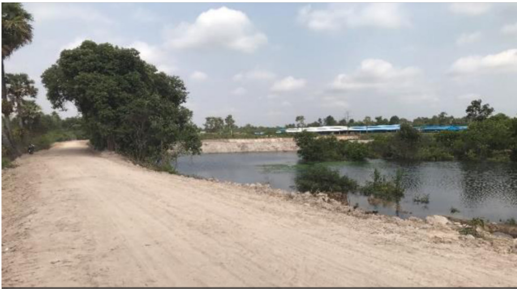
Dam renovation, at Chorm village, Chansor commune, Soth Nikom district in Siem Reap
