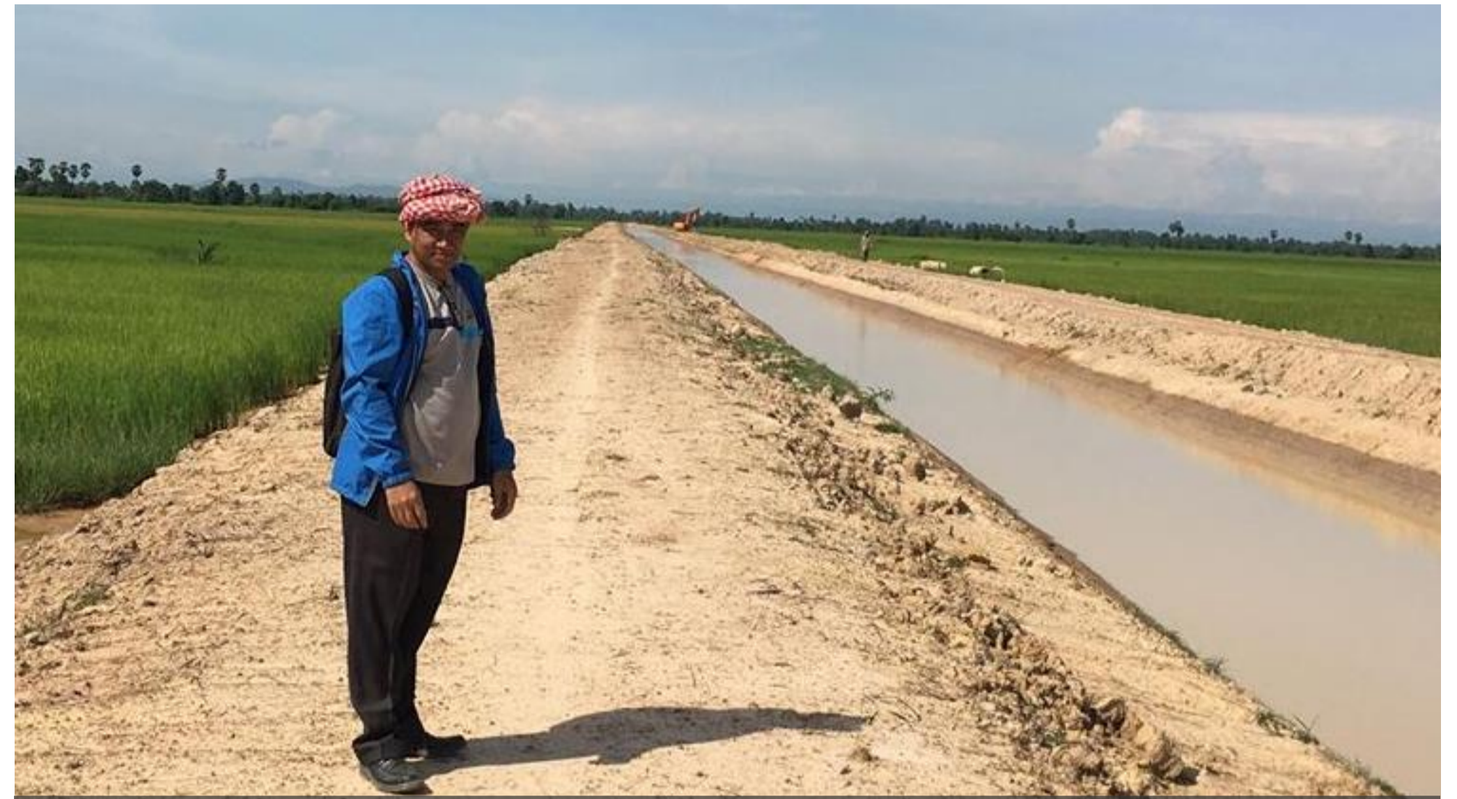
Irrigation canal renovation at Phteah Koh, Sre Sdok commune, Kandeng district in Pursat
